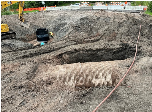
Condition of Previous CMP – note deformed top
