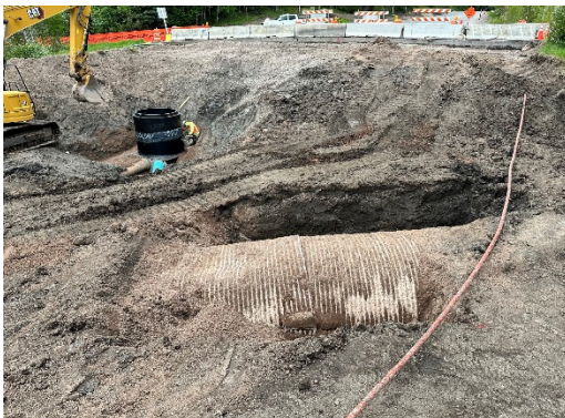
Condition of Previous CMP – note deformed top
